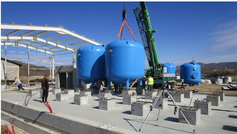
New water treatment plant (5'200 m3/d) in Trabotiviste
